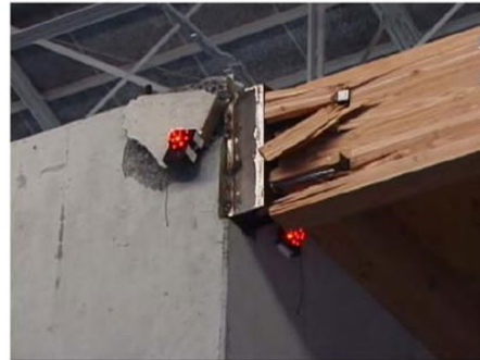
Fig. 19. Crushing of reinforced concrete and splitting of glulam timber beam
