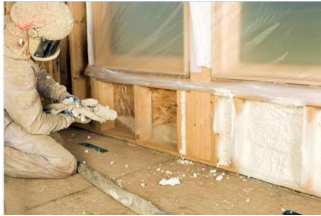
Figure 8 The process of insulating the walls with PUR foam blown with Forane™ FBA 1233zd
