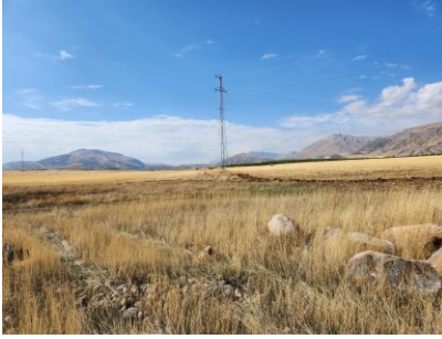
Photo 5 High Voltage Power Line passing through Parcel 1774
