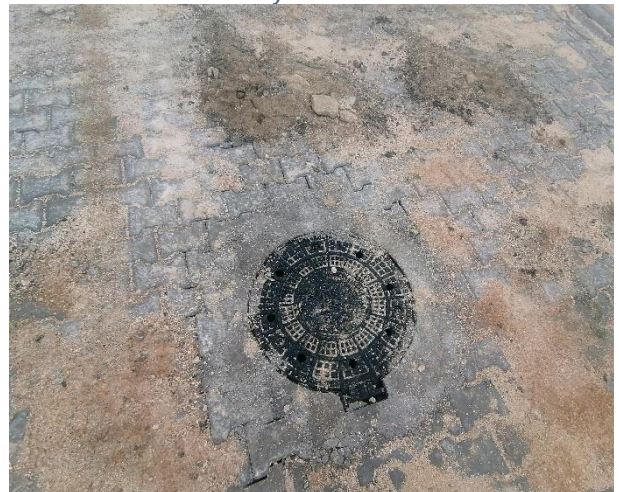
Photograph 43. Manhole in Resettlement Area (Infrastructure is available.)
