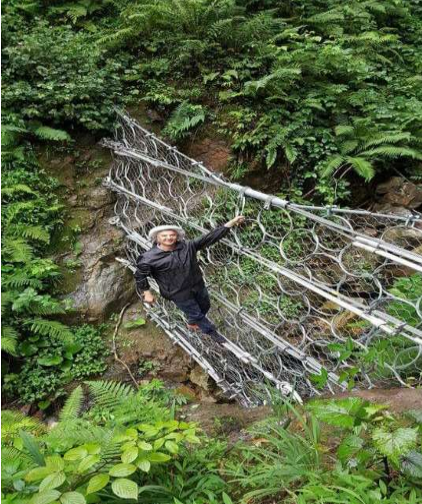
Steel-Mesh Debris Barrier (Güneysu – Rize)
