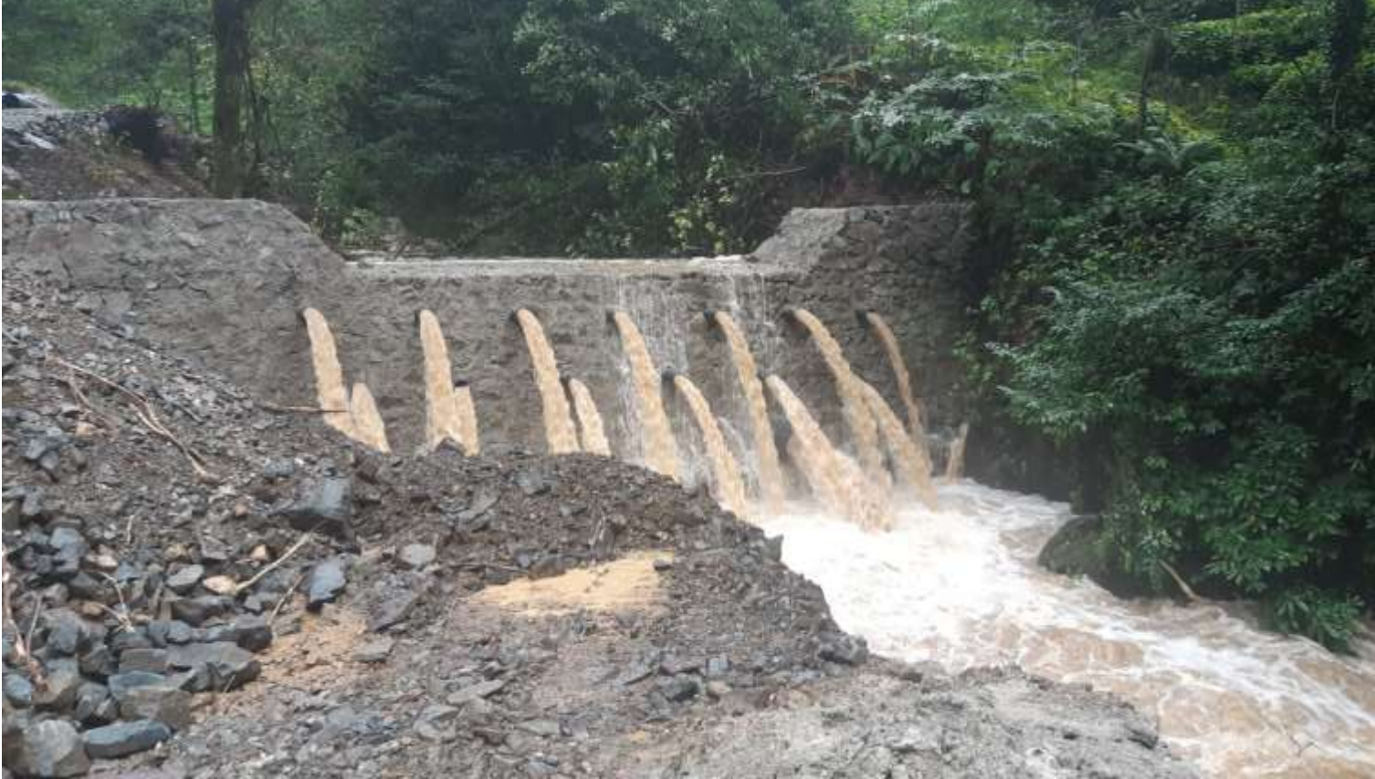
Ground Sills and Check Dams (Kalkandere - Rize)
